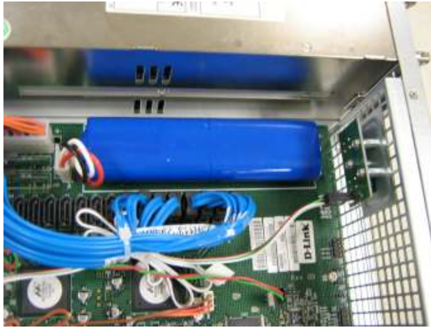
Figure 3-1 Battery Pack Installed on xStack Controller
