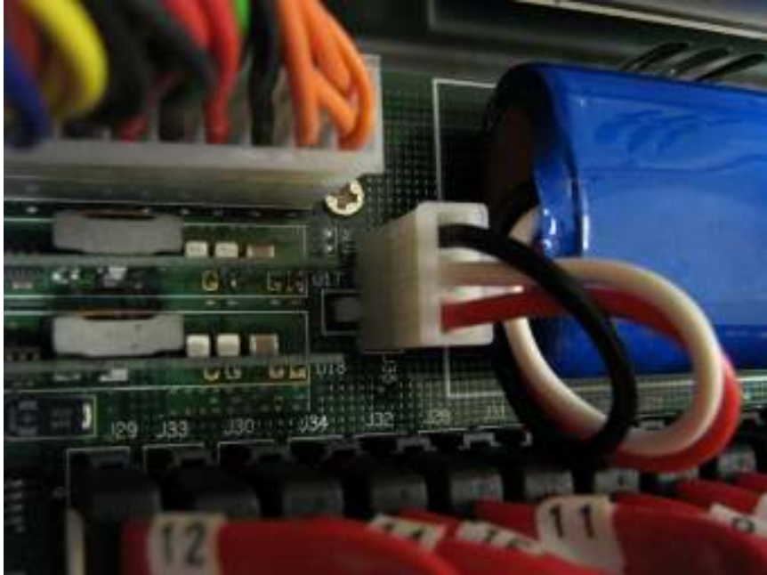
Figure D-4 Battery Plug Locked in Place
