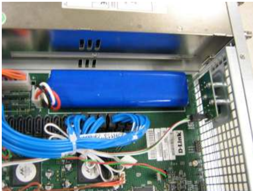
Figure D-5 The Installed Battery
